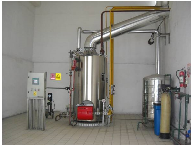
Figure 2: Methane Gas Boiler
